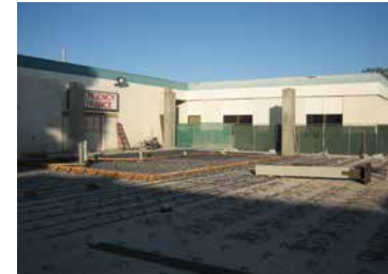
Beverly Hospital Central Plant
