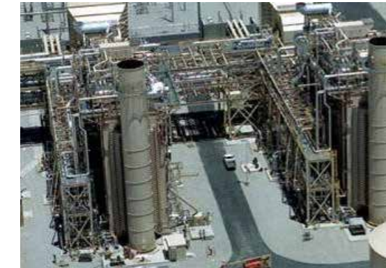
Elk Hills Power Plant Modifications
